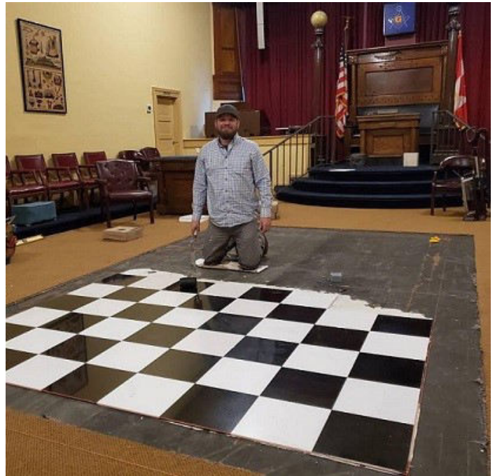
Above is EA Brother Kristian Nason, an operative as well as speculative Mason installing granite and marble tiles. The indented tessel will encompass the outside border. Photo from VW G. Winton Smith
